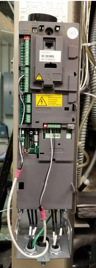
Figure 6: Actuators for Waterside Economizer
